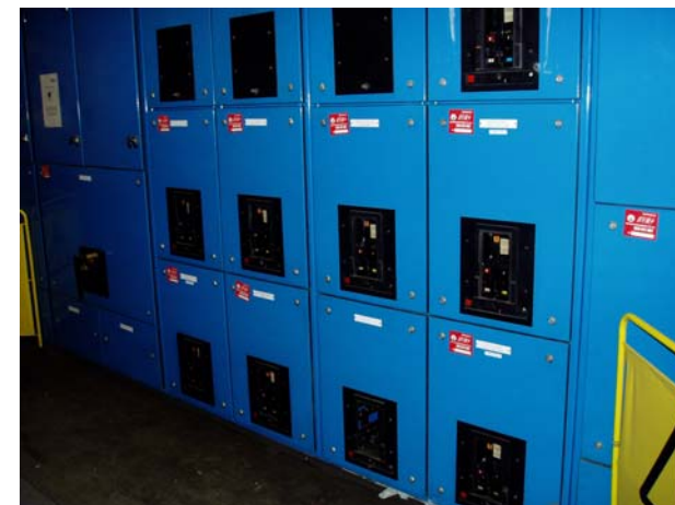
ACBs Merlin Gerin Selpact obsoletos
